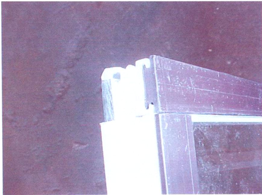
Magnetic Seal Surface of Storm Panel
